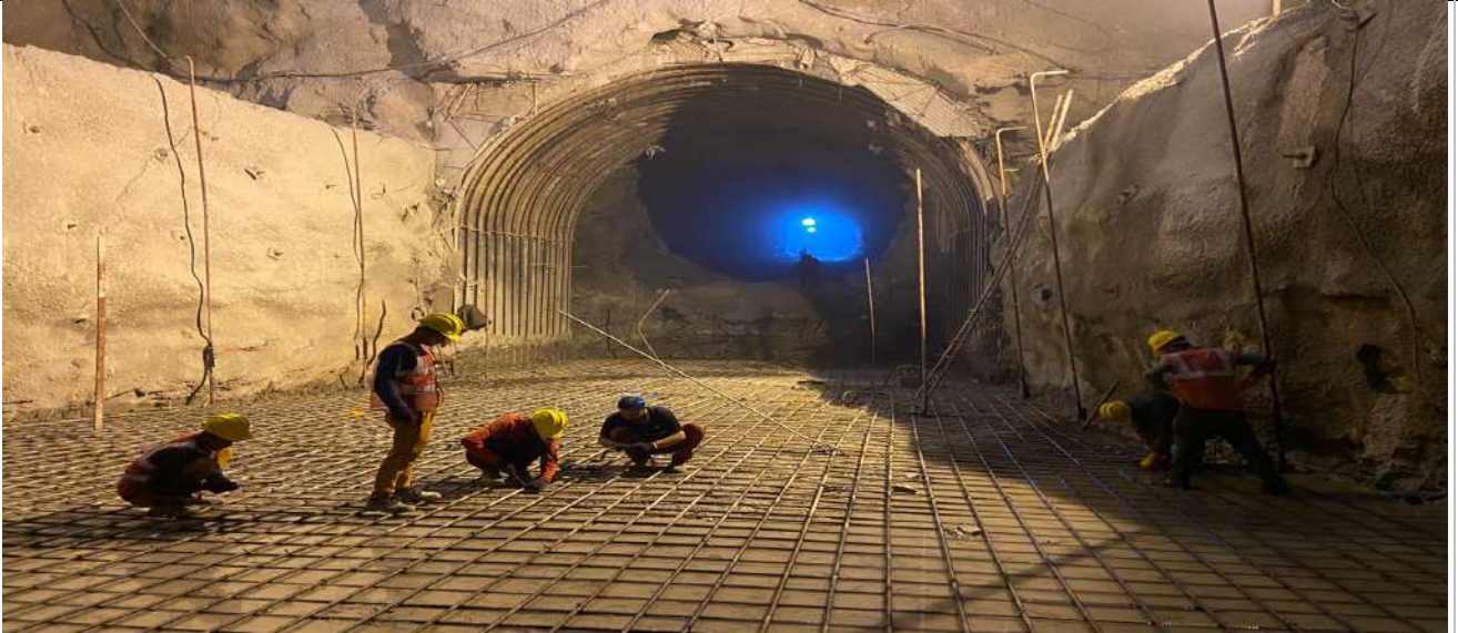
Excavation of TRT-1 Completed & through to Machine Hall. Raft Reinforcement of Draft Tube-1 at EL 1234.5M is in progress
