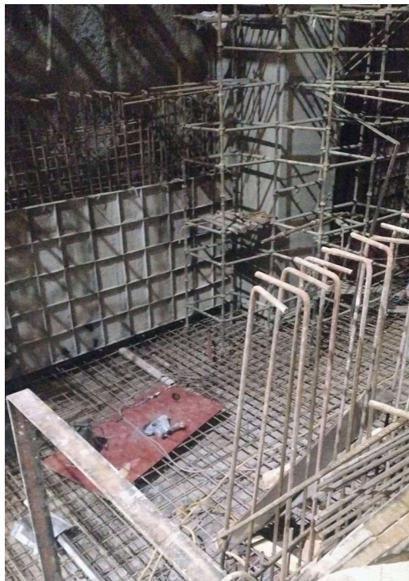
EARTH MAT AT SERVICE BAY
