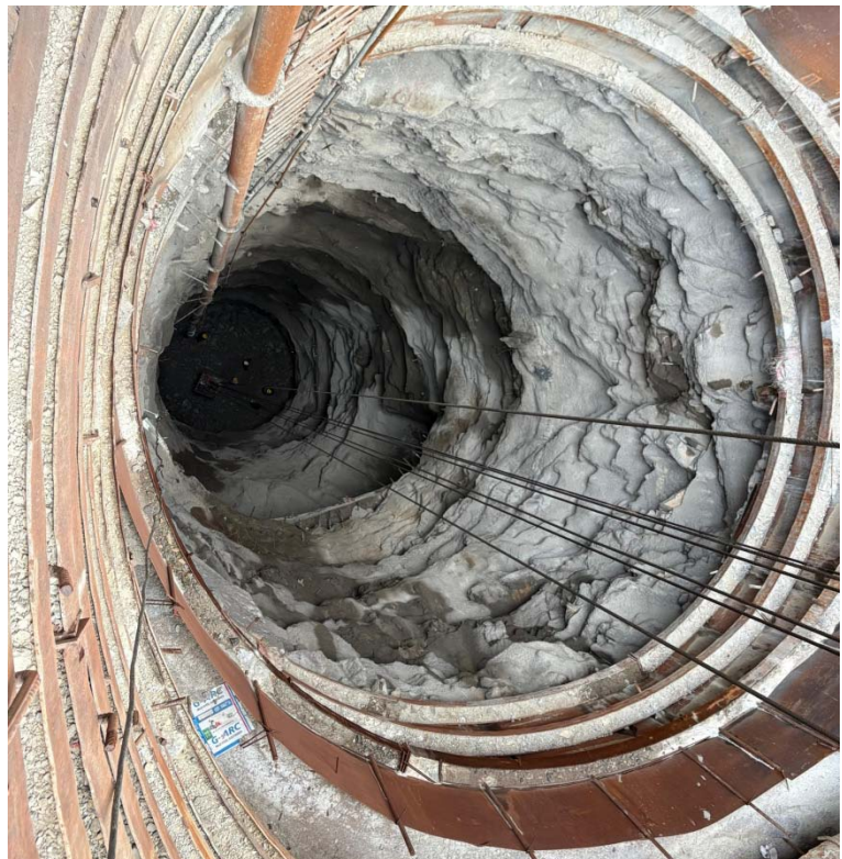
Vertical Pressure Shaft-3
