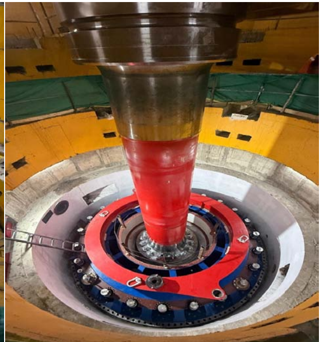
Unit# 1: Turbine Shaft
