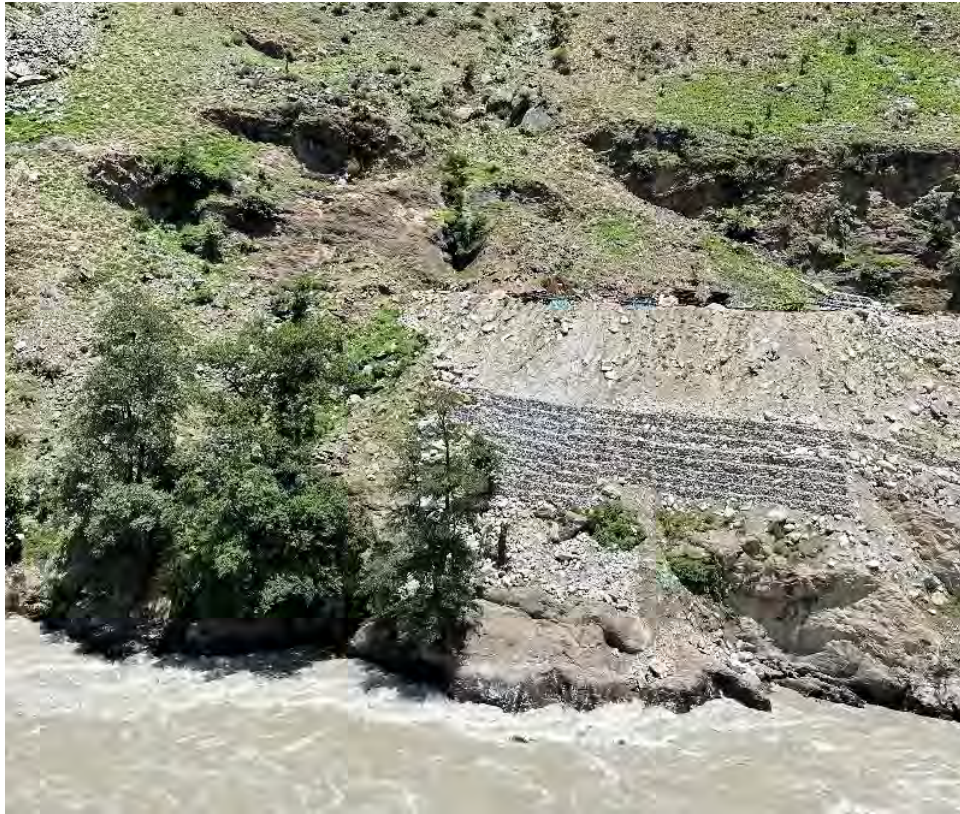
Photo 1. Toe wall constructed less than 30 m far from the HFL.
