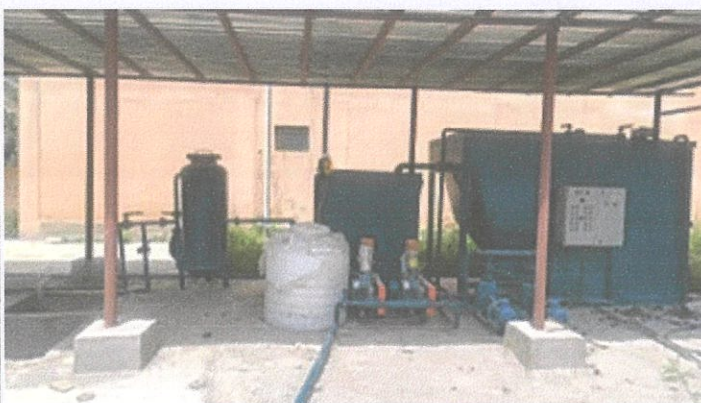
STP at Power House site
